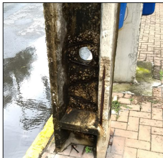
Figure 6. Corrosion of reinforcement with loss of concrete section.
