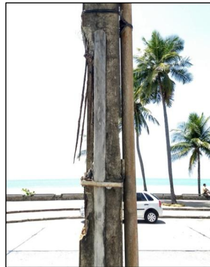
Figure 2. Post with broken reinforcement.
