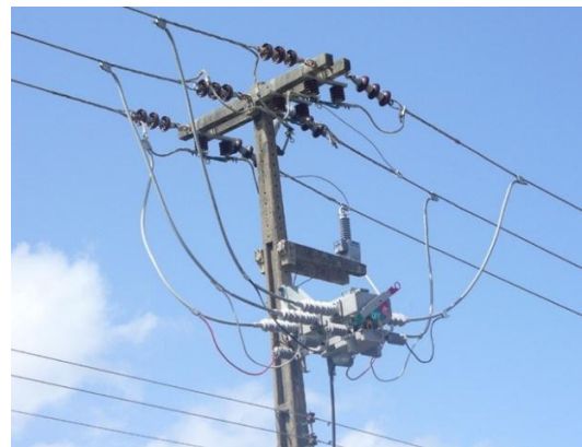
Figure 6. Example of coupler installation at an automatic switch.
