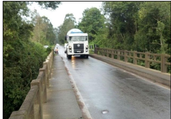
Figure 3. Traffic of heavy truck over an old-narrow bridge.
