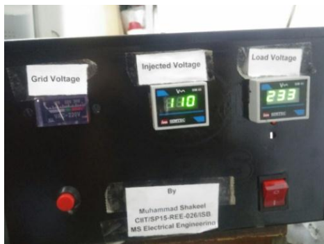
Figure 17. UPQC working at 50% Voltage Sag
