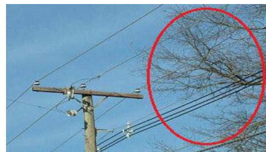
Figure (1): The possibility of connection of the distribution system conductors to a tree branch
